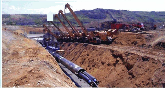
A typical view of the pipe pull-in operation showing the buoyancy system within the large diameter product pipe.
