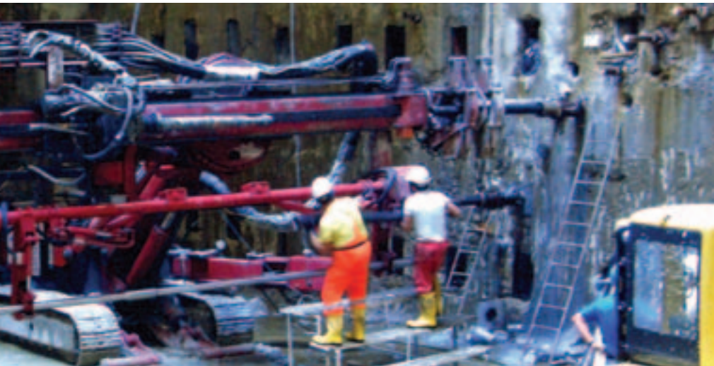
Drilling in progress on one of the galleries using the 10 t EGT rig with 2 m-long drill pipes that had been pre-built into 9 m lengths to save time in making connections to the probe
