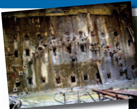
Above: the top half of one of the galleries before excavation with all but five of the holes in the section completed. These five are marked by square steel plates on the far left-hand side. The location of the sacrificial bore can just be seen in the centre of the gallery, about 1.5 m beneath the highest borehole
