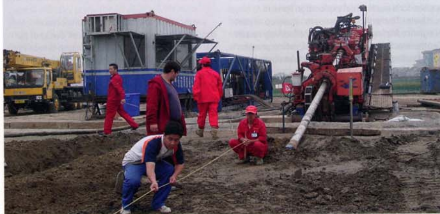
The guidance coil is straightened at the exit site in front of the 100t exit-side drilling rig
